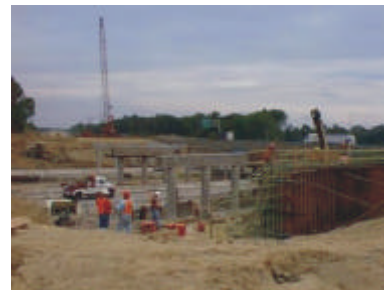
Ezicad will assist you to stake out pilings and foundations, and analyze design conformance
